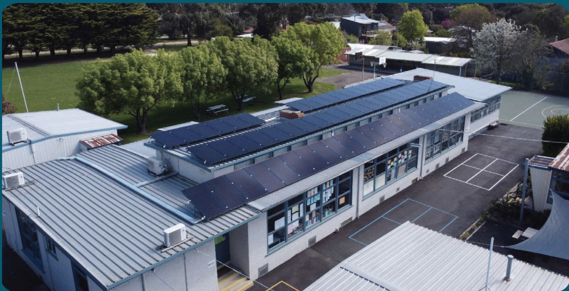
20kW solar system installed at Birregurra Primary School. Photo credit - Surf Coast Energy Group.
