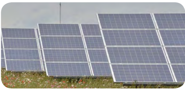
Westmill Solar Cooperative, UK. Courtesy of www.westmillsolar.coop .
